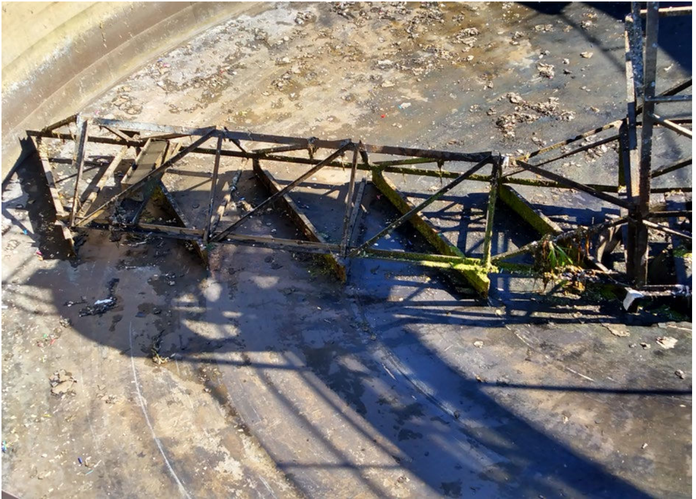
Photo #4 - Failed Sludge Thickening Equipment (Basin No. 2) Wastewater Treatment Plant City of Natchitoches, Louisiana
