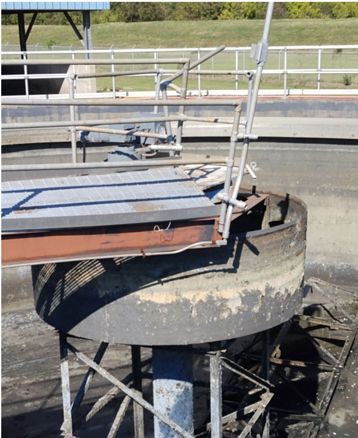
Photo #2 - Failed Sludge Thickening Equipment (Basin No. 2) Wastewater Treatment Plant City of Natchitoches, Louisiana
