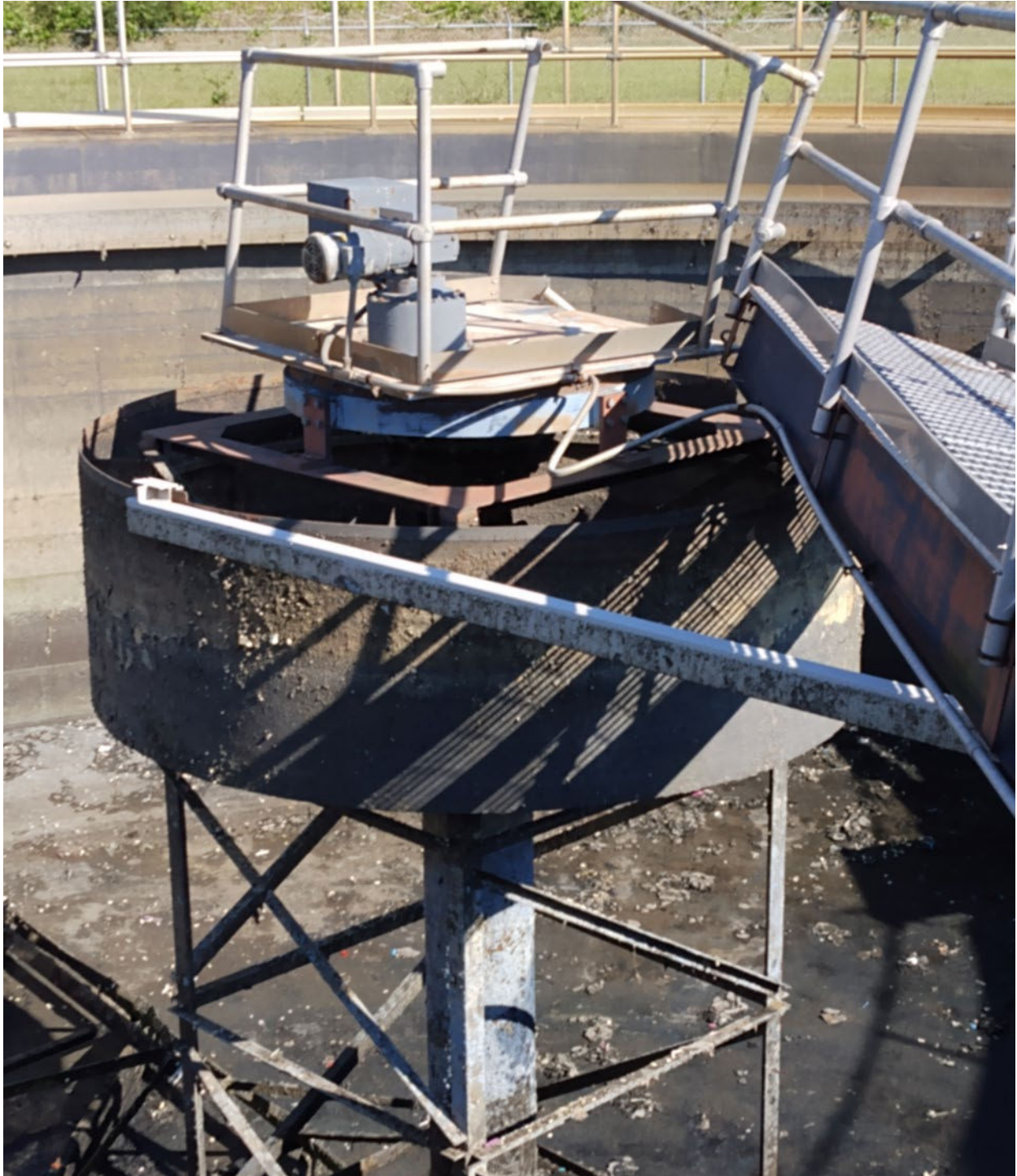
Photo #1 - Failed Sludge Thickening Equipment (Basin No. 2) Wastewater Treatment Plant City of Natchitoches, Louisiana
